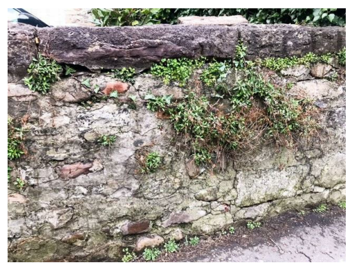
Further indication of plant growth that has penetrated the mortar joints in places
